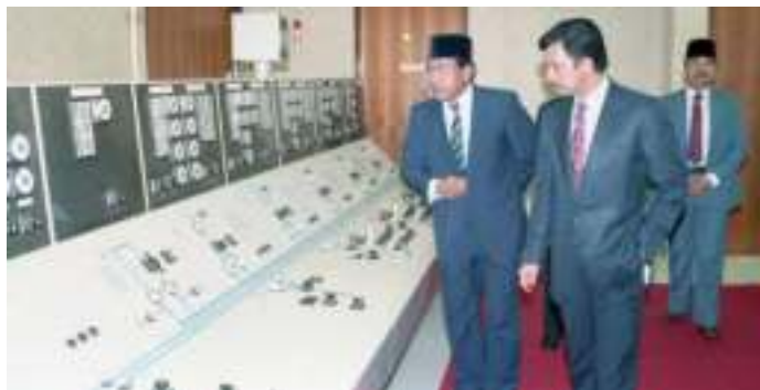
His Majesty the Sultan and Yang Di-Pertuan of Brunei Darussalam visited the Control Room at Lumut Power Station when it was launched in 1987
